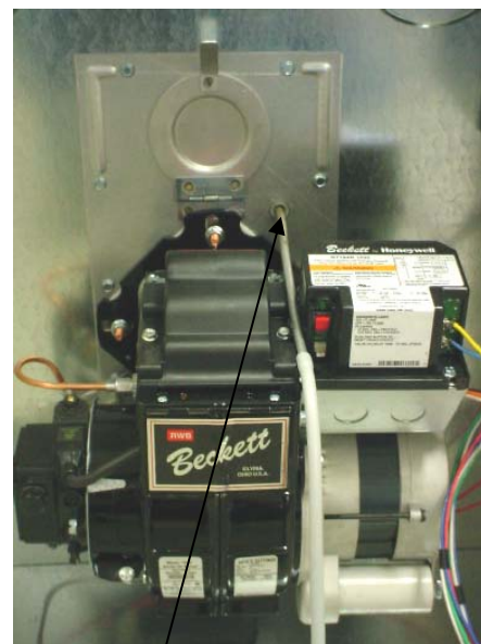
Over-fire draft access port.
